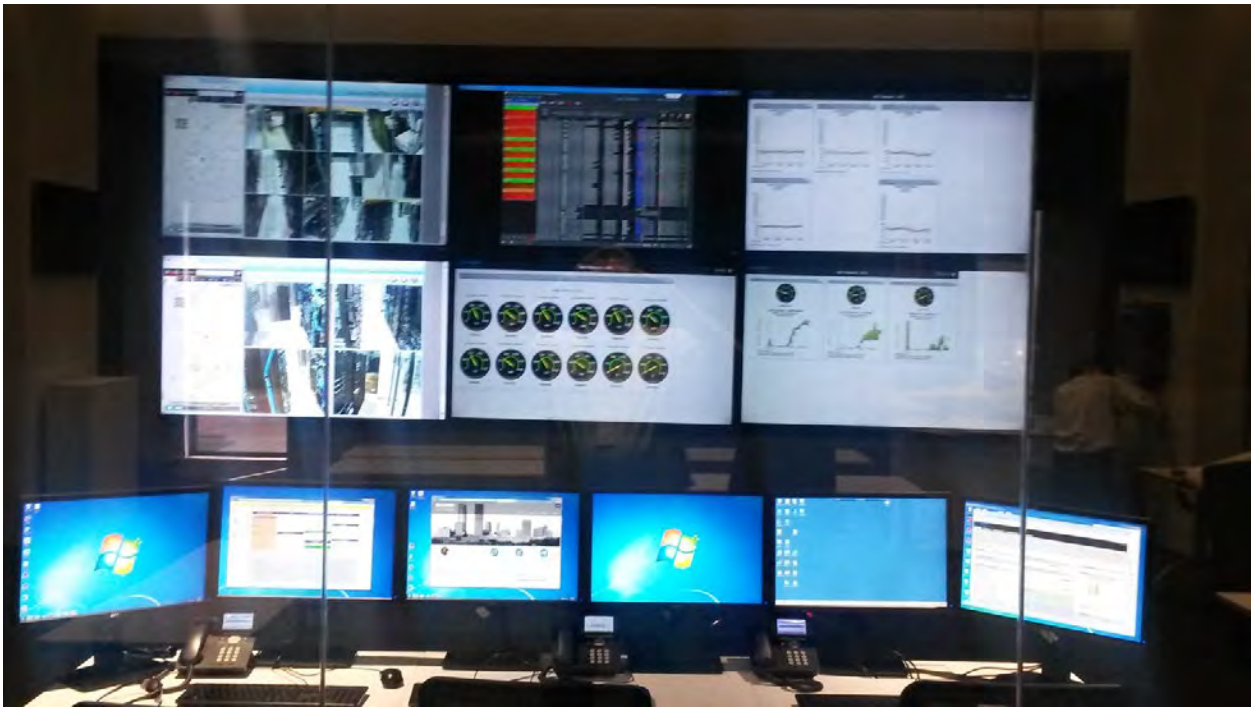
Securus Backup Network Operations Center
