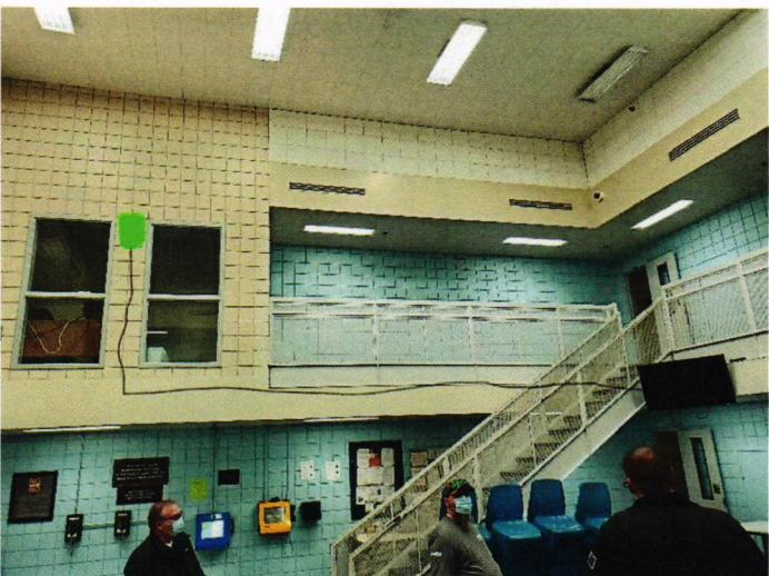
Unit 9100 WAP location and conduit run.
