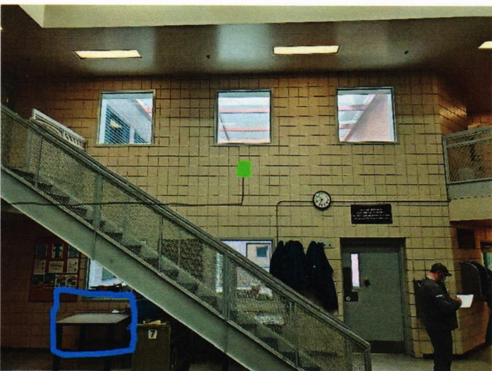
Unit 3100 WAP shown in green with conduit. Charging cart in blue. New power will be needed for the cart. 6 amps
