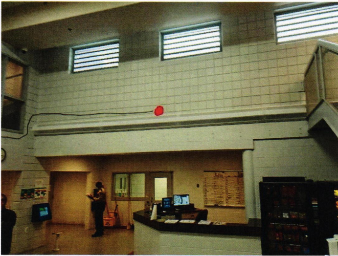
Unit 2100 conduit feed continued and WAP location,
