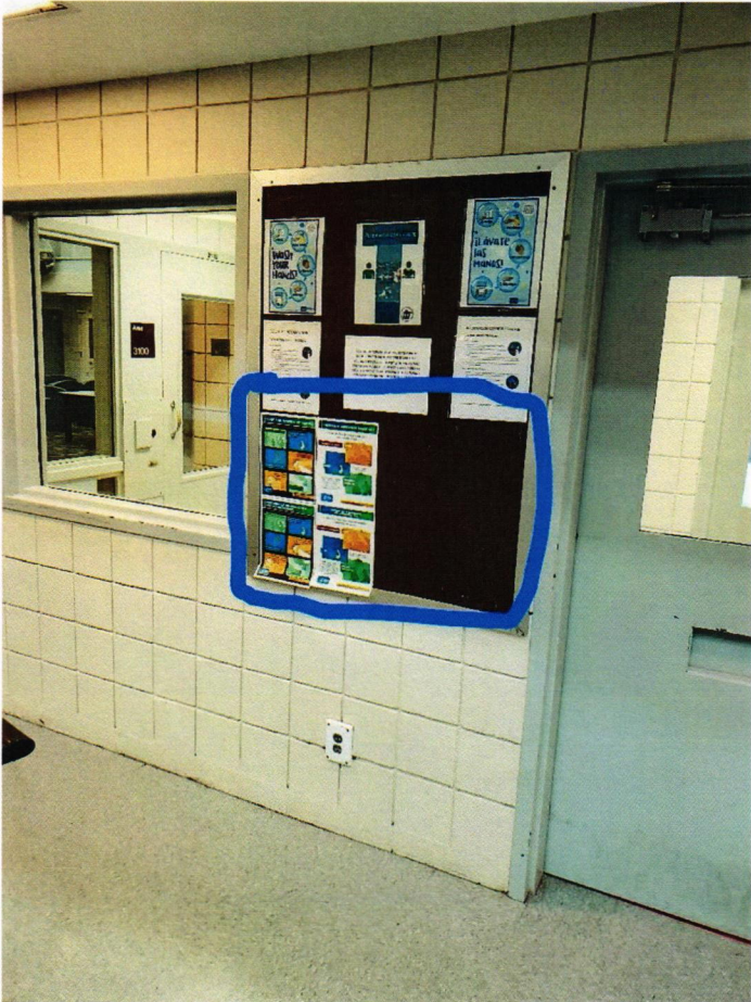
Unit 4100 charging cabinet. Bulletin board will be moved. Existing power will be used.
