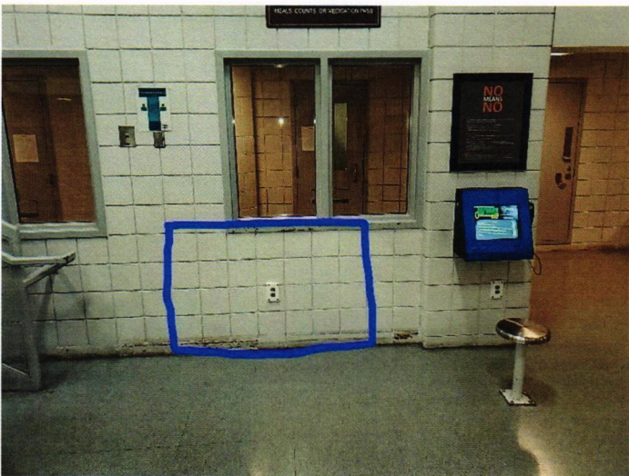
Proposed charging cart location using existing AC circuit if the circuit has 13 amps available. Otherwise, a new 20A circuit will be needed.
