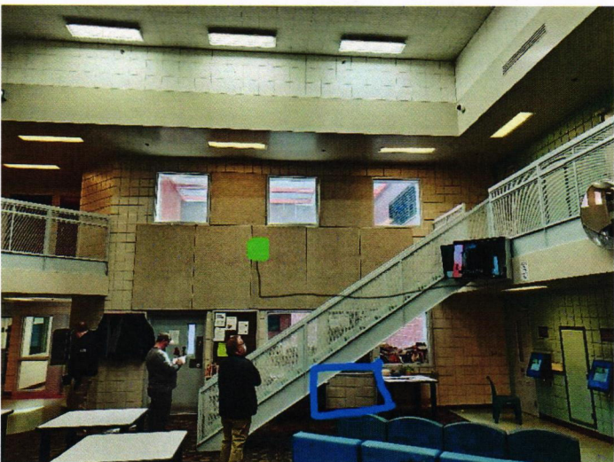
Unit 7100A WAP and conduit run. Charging cart is in blue. The cart requires 13 amps, so new power may be needed.
